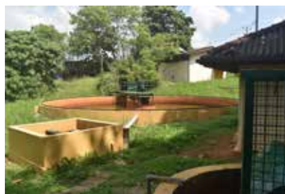
Waste water treatment plant
